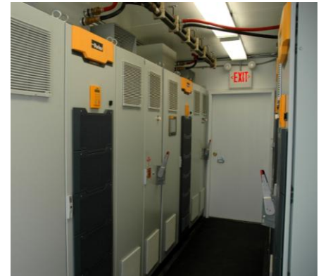
Interior view of 4 Megawatt container
